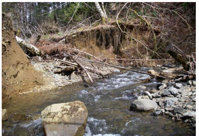
Upstream view of actively eroding bank near the end of the survey.
