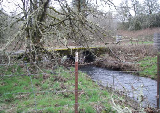
Unit 1 - A downstream view of the Foster Creek Upper survey start. Triple culvert crossing here.
