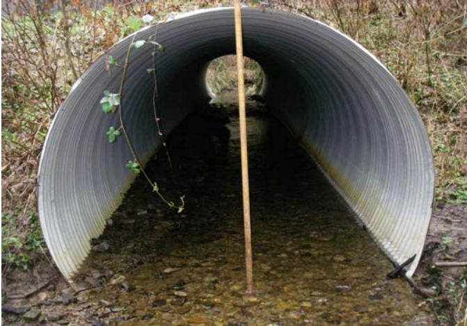
Unit 1 - Downstream view of culvert at start of survey. Wolf Cabin Creek Road crosses here.
