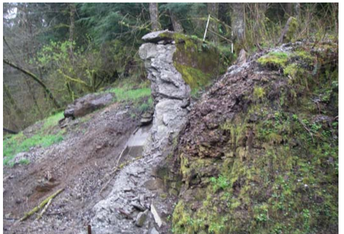
Unit 35 - right side of old, dismantled dam near the end of the survey.
