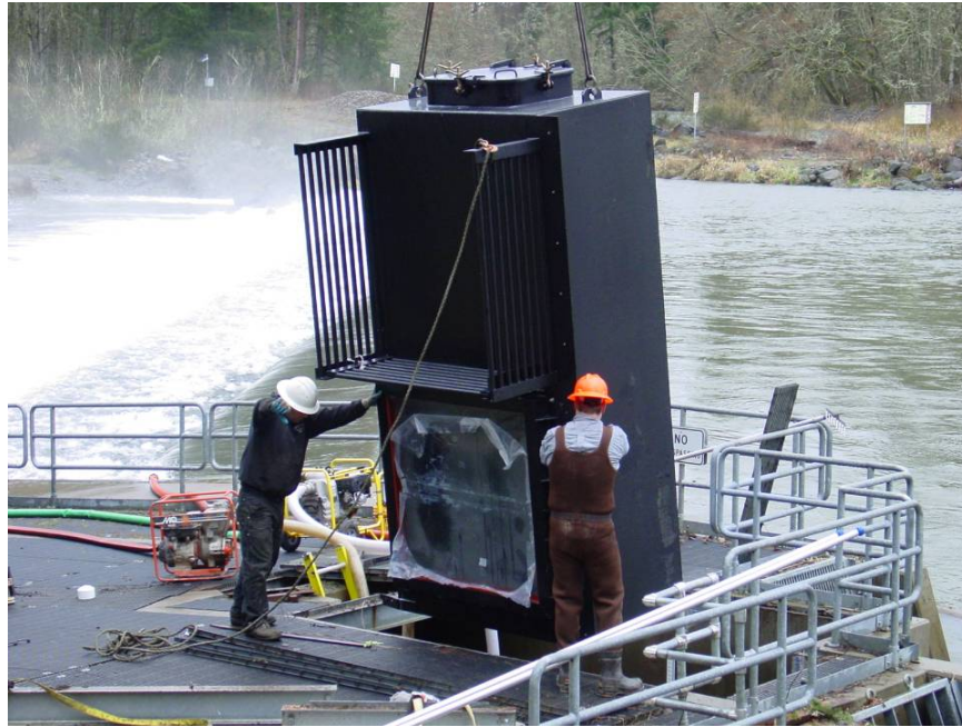
Figure 7. Installation of housing vault at Upper Bennett Dam fishway for video recording system to monitor fish passage.
